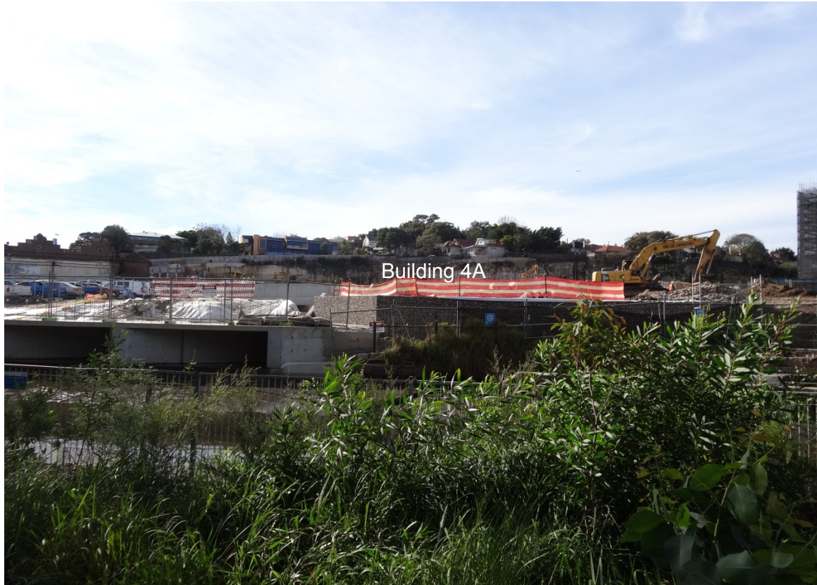
Figure 3: Looking east from The Crescent across the Harold Park site towards the cliff face and proposed Building 4A location
