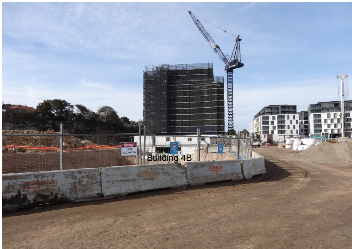
Figure 6: View of Building 4B location, looking south towards Precinct 2 buildings currently under construction (L) and the complete Precinct 1 buildings (R)
